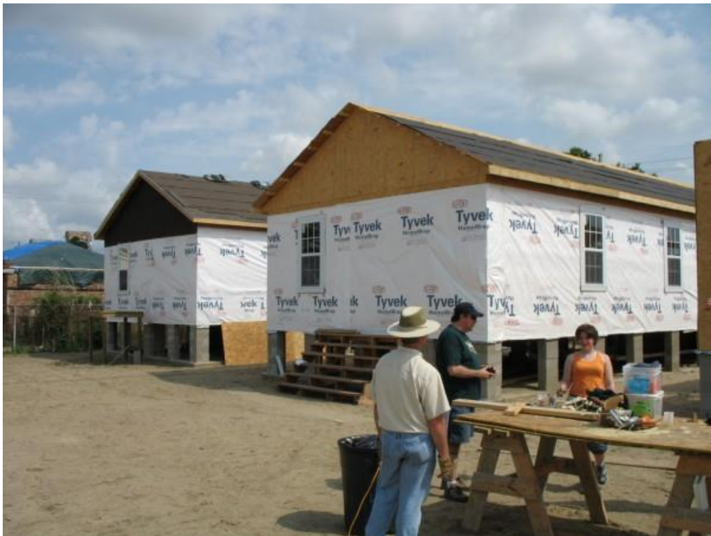
First 3 houses built in New Orleans after Katrina, built by Habitat for Humanity, worked on by the AE club.
